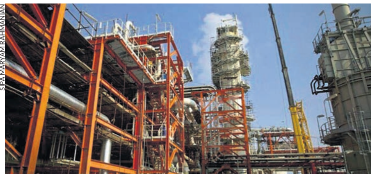
Les installations du champ gazier North Field.
